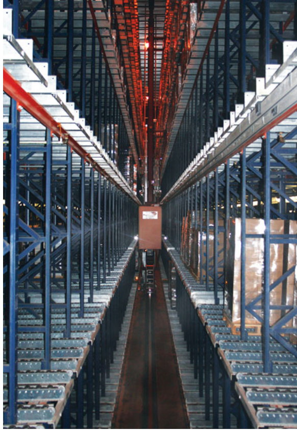
Fig. 10.12 Multiple story storage/retrieval system capable of moving product into and out of storage by computer-controlled vehicles (courtesy of Westphalia Technologies, Inc., York, PA)
