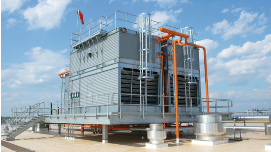
Fig. 7.28 Field installation of an evaporative condenser on an industrial ammonia refrigeration system (courtesy of Baltimore Air Coil, Jessup, MD)
