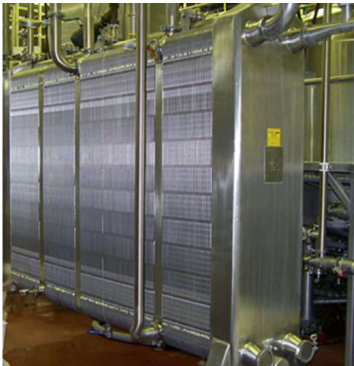
Fig. 5.5 A plate heat exchanger used for cooling of mixes following batch pasteurization. This also provides a good illustration of plate heat exchangers used for HTST pasteurization, when properly configured
